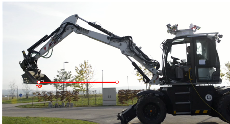
Figure 1: Our test vehicle in Renningen with an example trajectory to be followed. More info on https://www.bosch.com/stories/learning-control-for-advanced-excavator-assistance-functions/ .
